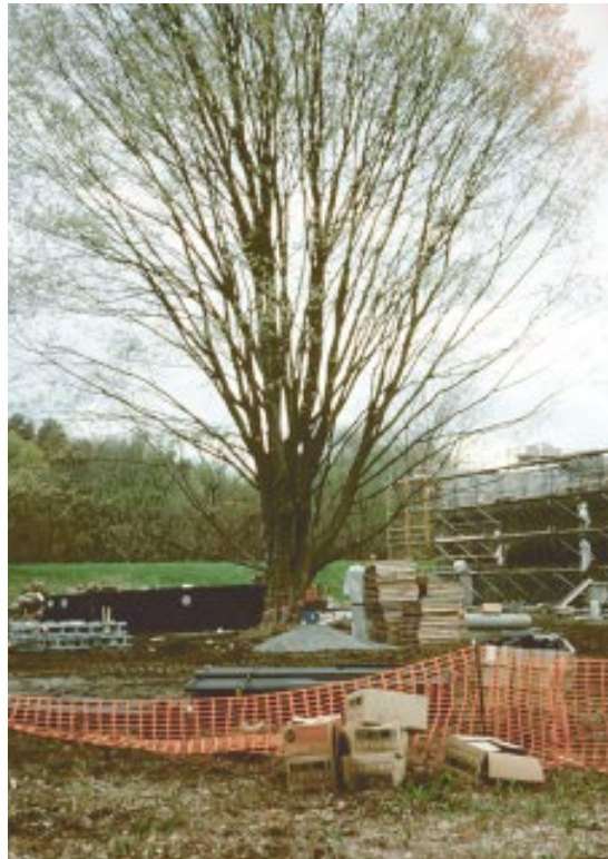
Figure 5. Although the root zone of this tree was defined with snow fencing, lack of adequate site supervision made that a wasted effort (top). The broken limb and damaged bark on the tree at bottom are the most visible injuries, but the excavated material piled beneath it will soon suffocate the roots.
