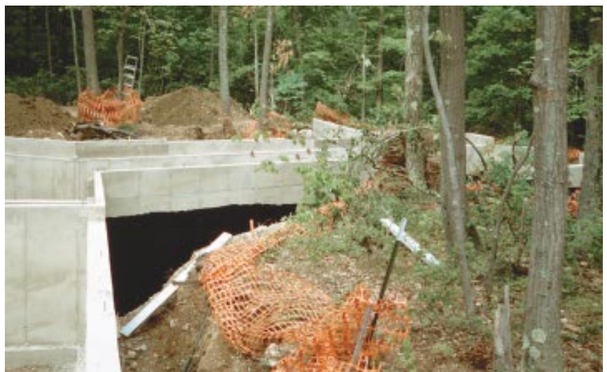
Figure 3. Don't try to save trees that can't be saved. The oaks at the edge of this foundation have lost too many of their roots to survive for more than a few years. It would have been cheaper and much less troublesome to remove them before starting to build.
