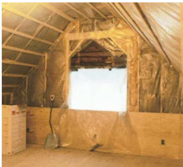
Figure 6. Prepped for finishes, the new attic room has straight ceiling lines, a level floor, and a much stronger roof. Along the bottom of the walls, plywood provides solid nailing for paneled wainscoting.
