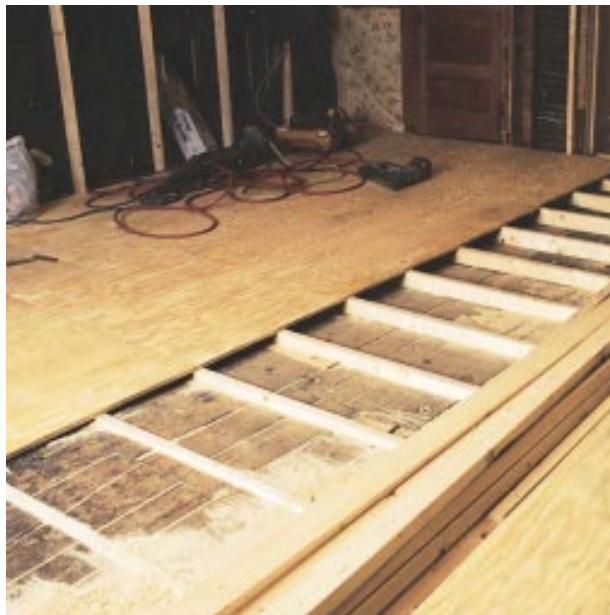
Figure 5. A new \frac{3}{4} -inch tongue-and-groove plywood subfloor provided a sound base for carpet and built-ins.
