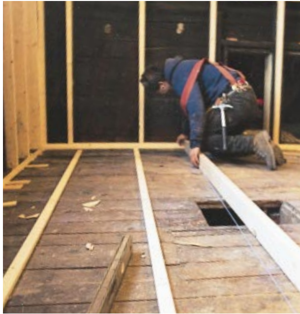
Figure 4. After installing a level nailing strip around the perimeter of the room, the author snapped cut lines on each sleeper. This scribed sleeper system leveled and took the sags out of the floor.
