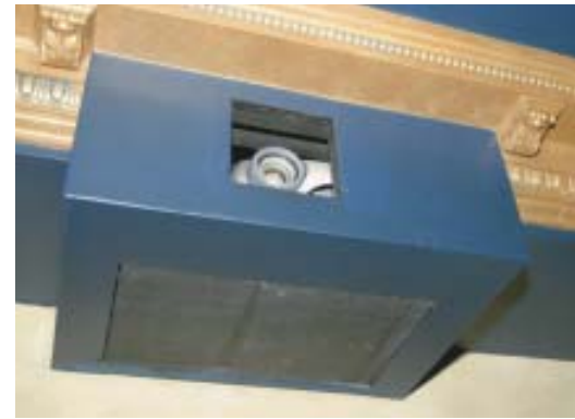
Figure 10. Projectors are noisy, so they're typically placed in soundproof enclosures. This unit projects through a piece of glass and can be serviced through the access panel below. The box is mechanically vented through the soffit to prevent the projector from overheating.
