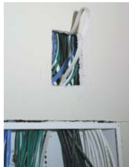
Figure 5. The electrician ran this Romex when no one was looking. It shouldn’t be in with the A/V cables and will cause interference if it’s not removed and brought in separately from below.
